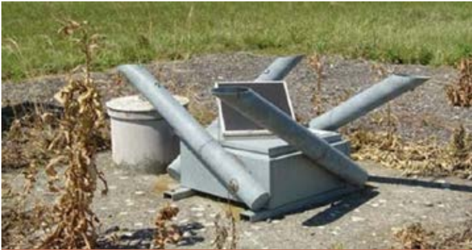
An underground stationary gas powered noise generator
