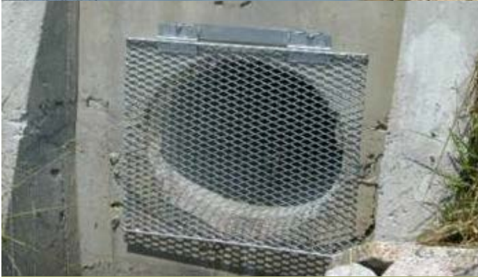
Floating balls and bird netting to cover the water, and drainage opening protection
